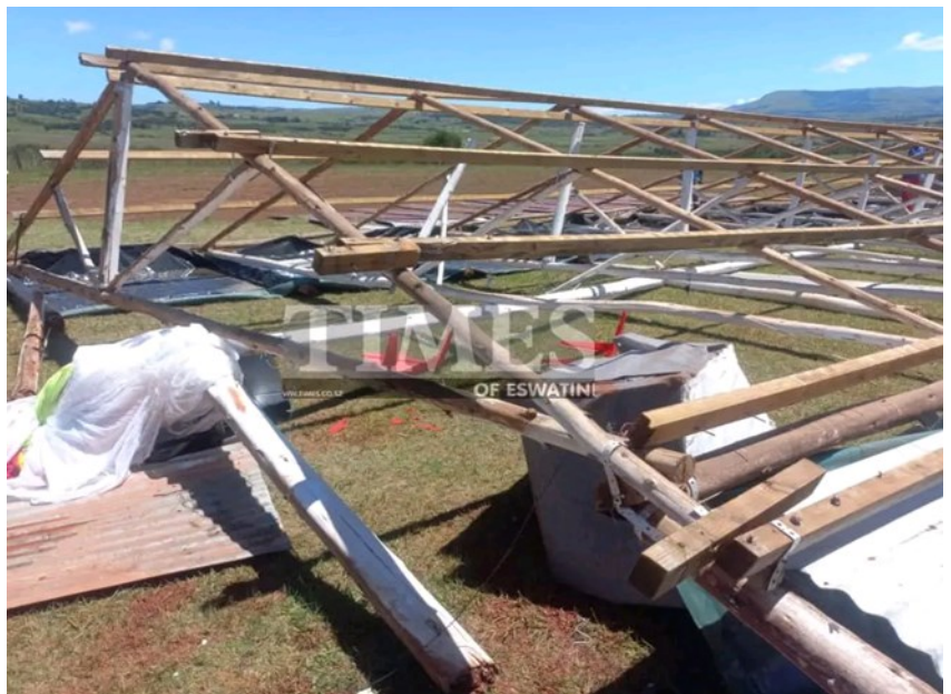
Roof that was blown down by strong winds that accompanied severe thunderstorms in June, courtesy of Times of Eswatini
